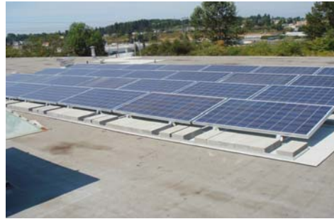
Solar arrays on the roof of the JATC building, put up by the fifth year class.
