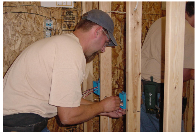
Ben Doyle racing to complete his residential project for the Western States Electrical Contest held in Boise, Idaho.
